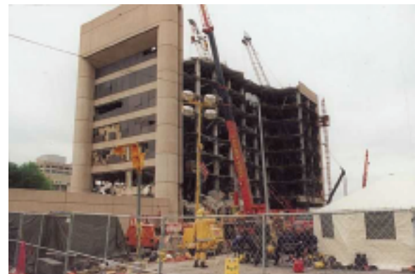
Alfred P. Murrah Federal Building after bombing attack. Photo by Oklahoma City Police Department
